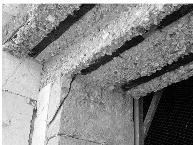
FIG. 10 - Limestone cracking provoked by the replacement of a wood lintel by a reinforced concrete lintel in the Governor's Palace, next to the House of Turtles (Uxmal).
