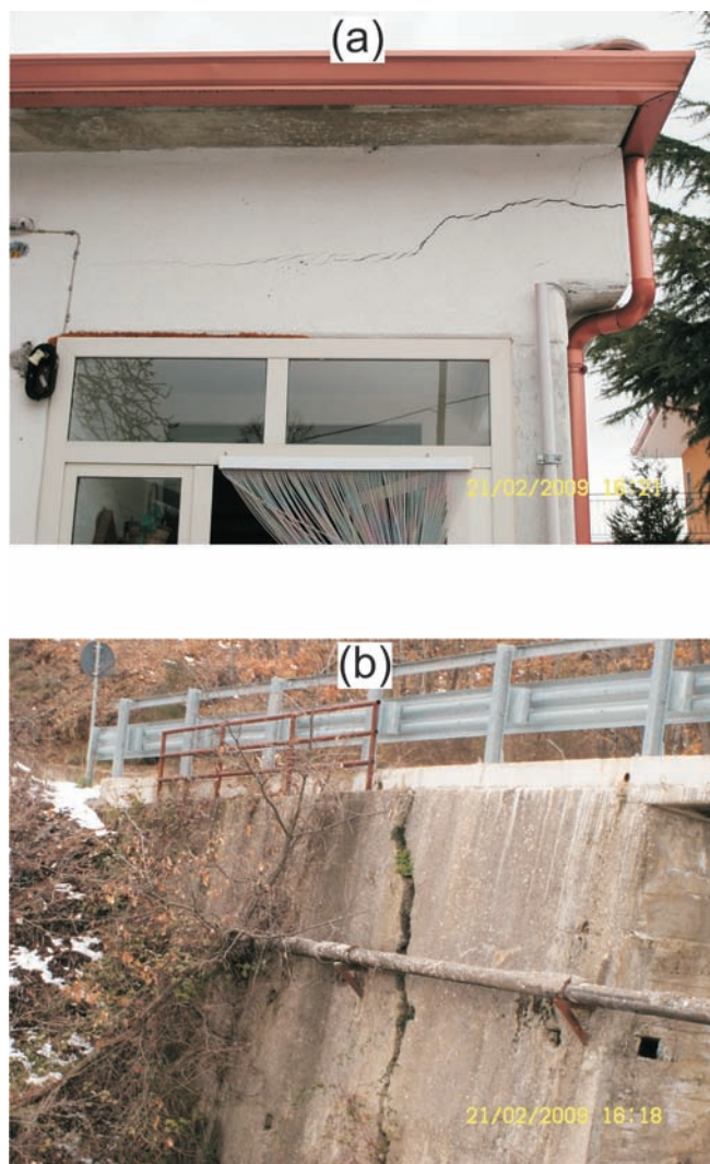
FIG. 5 - Examples of damages to infrastructures recognized above the Pietra Maura landslide body: a) Cracked building; b) Main road cracked bridge.
