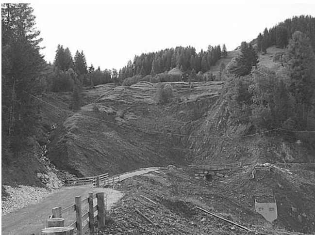
FIG. 15 - The Col da Oi landslide which affected a bridge on the road leading to the hamlet of Costa.
