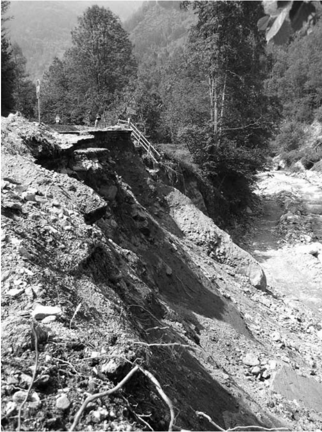
FIG. 6 - Intense bank erosion involving the provincial road near the junction of the road leading to Salza di Pinerolo and Massello.
