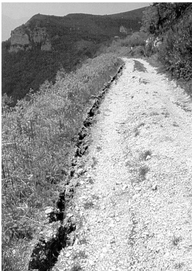
FIG. 3 - Example of a non-catastrophic failure along a discontinuity in the soil cover.
