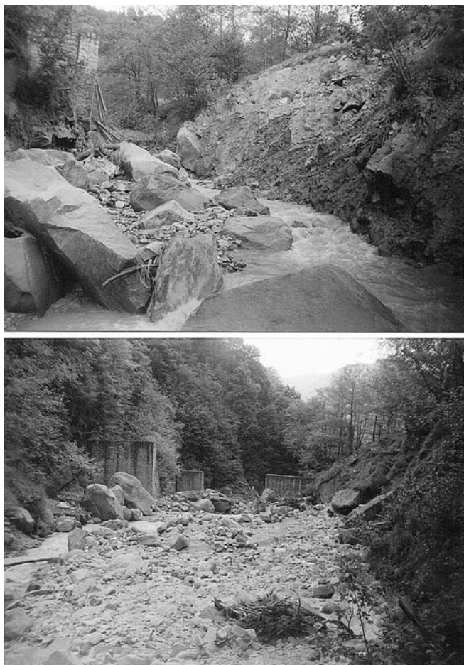
FIG. 8 - Rainfall prior to the Sâmbăta valley (upper photo: the hydrometric station, destroyed; lower photo: the dam upstream the resort).
