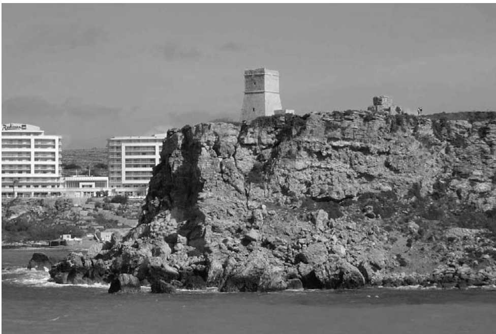
FIG. 4 - The coastal tower overlooking Ghajn Tuffieha Bay was built for defence purposes in 1637 by Grand Master Lascaris. The deep fracture within the Upper Coralline Limestone plateau is putting the historical tower at risk due to the retreating cliff.
