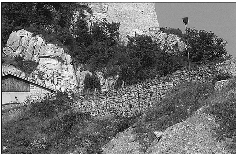
FIG. 6 - The gabion wall affected by gully erosion.
