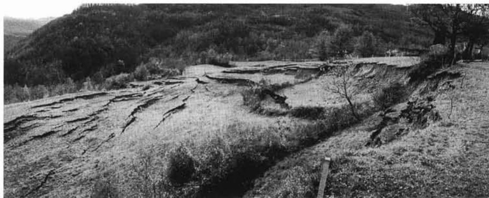
FIG. 6 - The crown and the head of the reactivation of the Sivizzo landslide occurred in November 2000.
