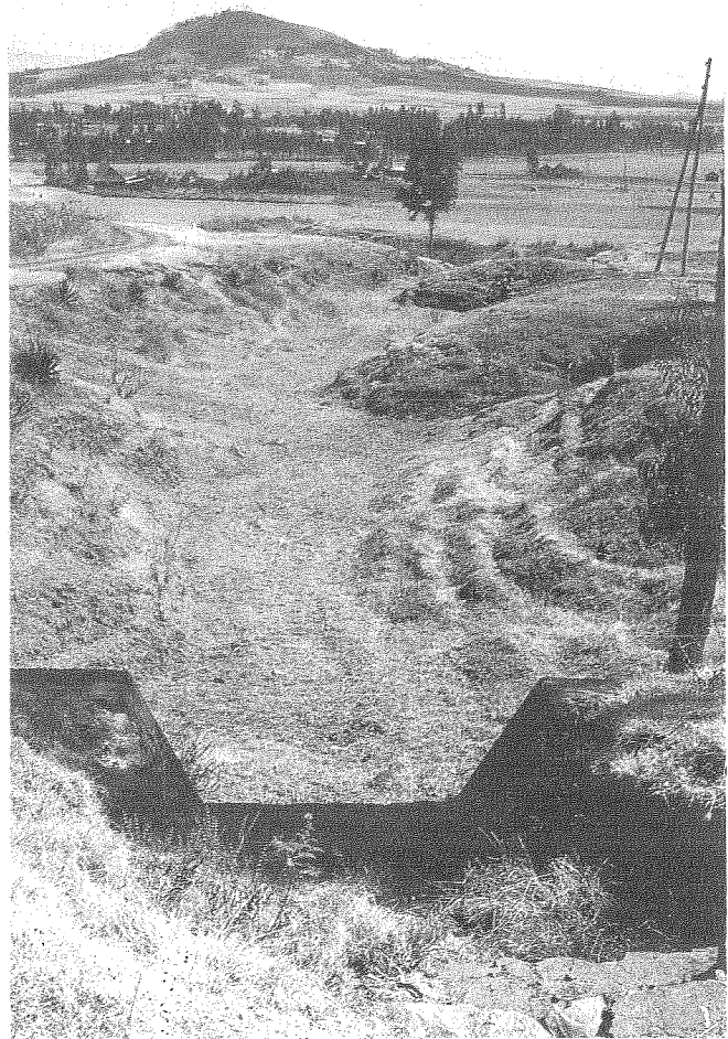
FIG. 6 - To minimize the undercutting, sills are constructed. Gullies are here deep and gradually become shallower and disappear downslope.
