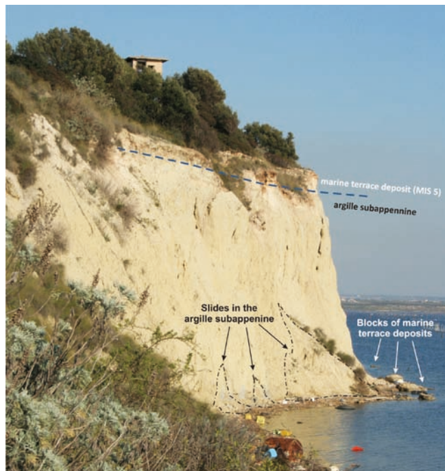
FIG. 2 - Present-day cliffs in the Mar Piccolo on the east side of Punta Penne (B in fig. 1). The sharp contact between the argille subappennine and the overlying Tyrrhenian (MIS 5e) calcarenites is shown. Present-day erosion induces rock falls in the Tyrrhenian calcarenites and slides in the argille subappennine unit.
